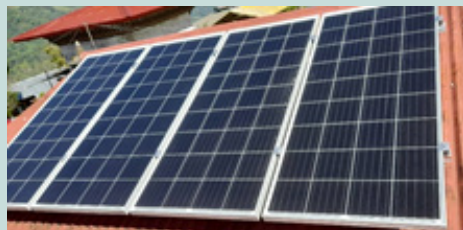
Figure 17: Solar Panel and array
