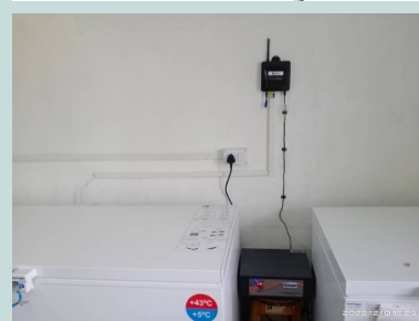
Figure 21: RTMD to remotely monitor the temperature of vaccine in the refrigerator
