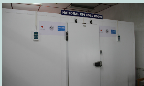
Figure 9: Walk-in-Cooler to store large volume of vaccines at positive temperature
